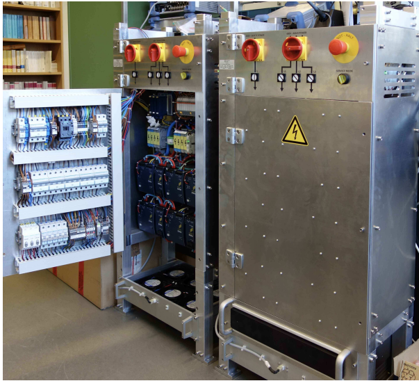
FIG. 6.2 – Two safety and power cabinets under 24/7 testing before installation into the camera.
